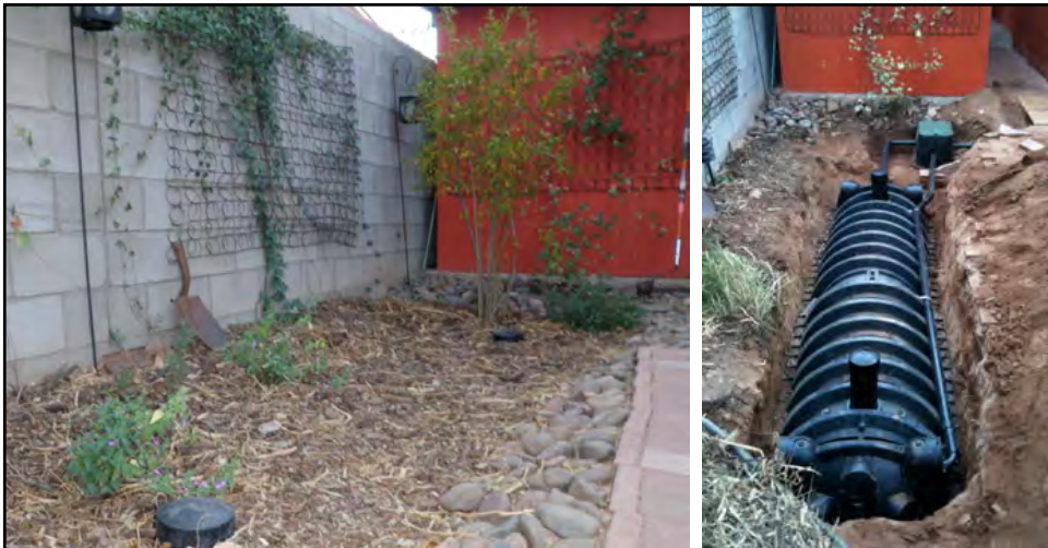
Infiltration chambers used for sub-surface kitchen sink greywater discharge
