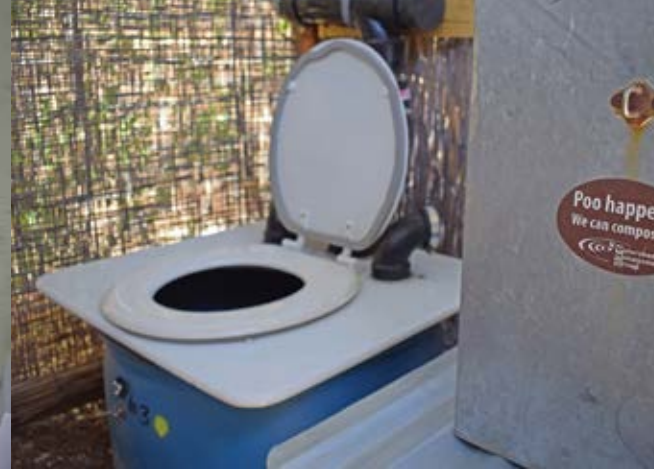
Barrel composting toilet
