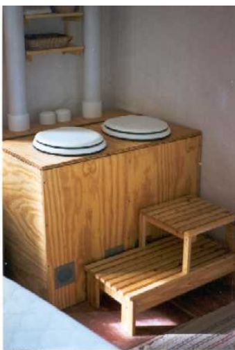
Indoor composting toilet
