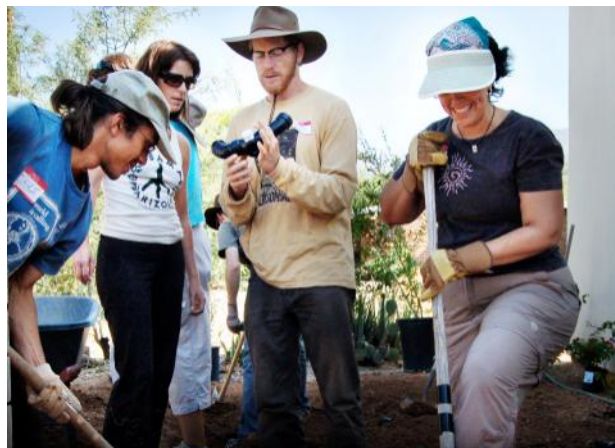
Brad Lancaster, one of WMG's certification instructors, teaches how to install a branched-drain greywater system.
