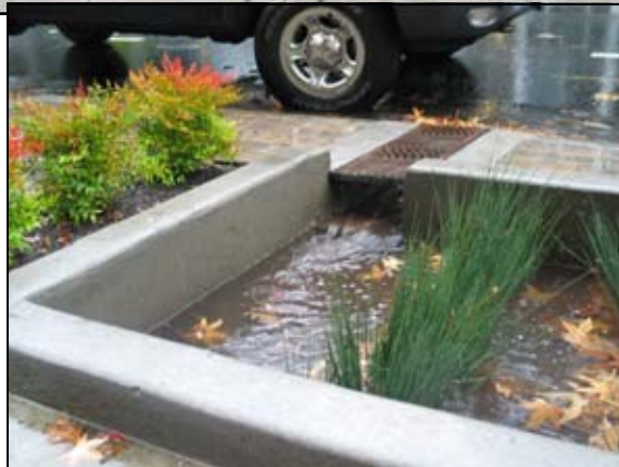
Portland Green Street facilities collect stormwater from the street and sidewalk into the vegetated area. Photos courtesy Dave Elkin, Portland Bureau of Environmental Services.
