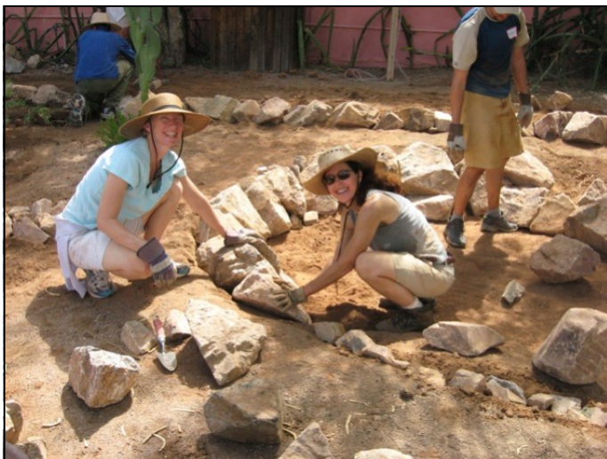
Volunteers help install water harvesting berms in the Grant Campbell neighborhood in Tucson as part of a larger effort to green their neighborhood.
