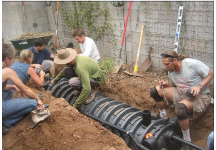
WMG Certification students learn how to install a kitchen resource drain with an underground infiltration chamber.
