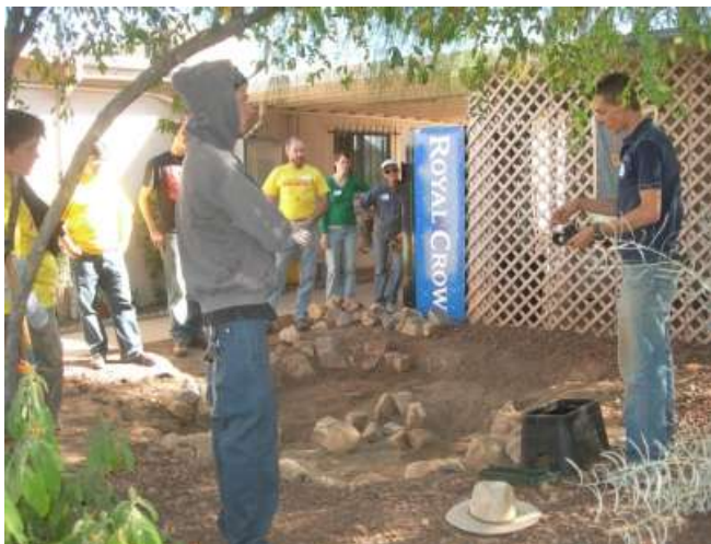
Catlow Shipek instructing students and teacher from Sky Island how to install a greywater system at Casa Paloma - housing for homeless women.
